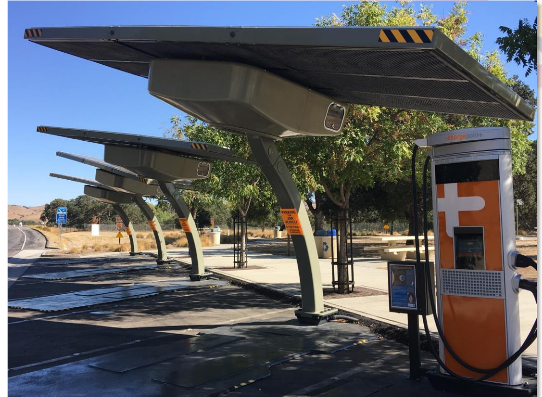
Fully solar-powered EV charging station deployed for CALtrans.
