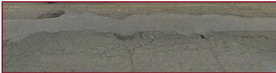
Figure 8. Poor Pavement Condition on Service Road
