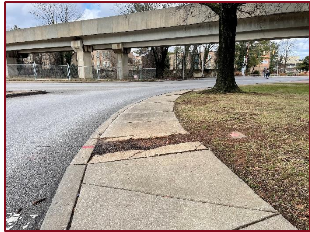
Figure 3. Inaccessible Sidewalk Conditions on Wabash Avenue
